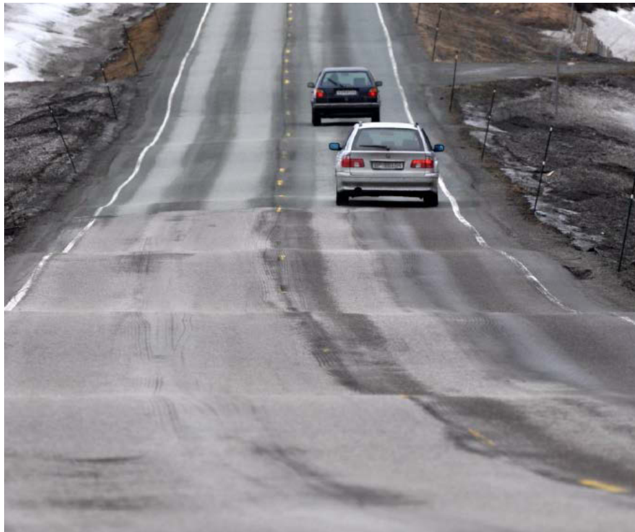
Figure 2. Frost-heave pavement damage in Norway (Ystenes 2011)
